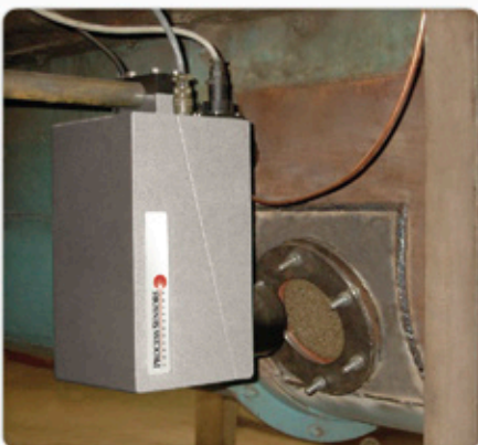
Moisture through sight glass
